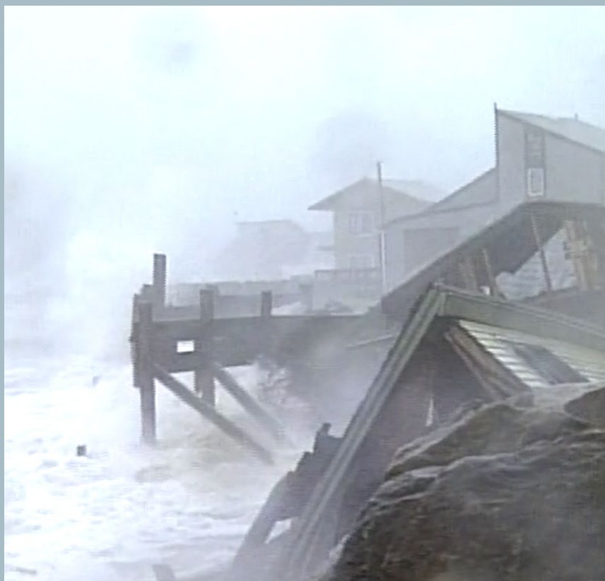
Damage in Maine from Hurricane Bob in 1991, the last Category 2 hurricane to make landfall on Maine's coast. © WGME
