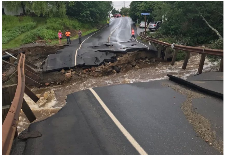
Culverts washed out along Route 186 in the Village of Birch Harbor during a flooding event on June 9, 2021. © Dale Church
