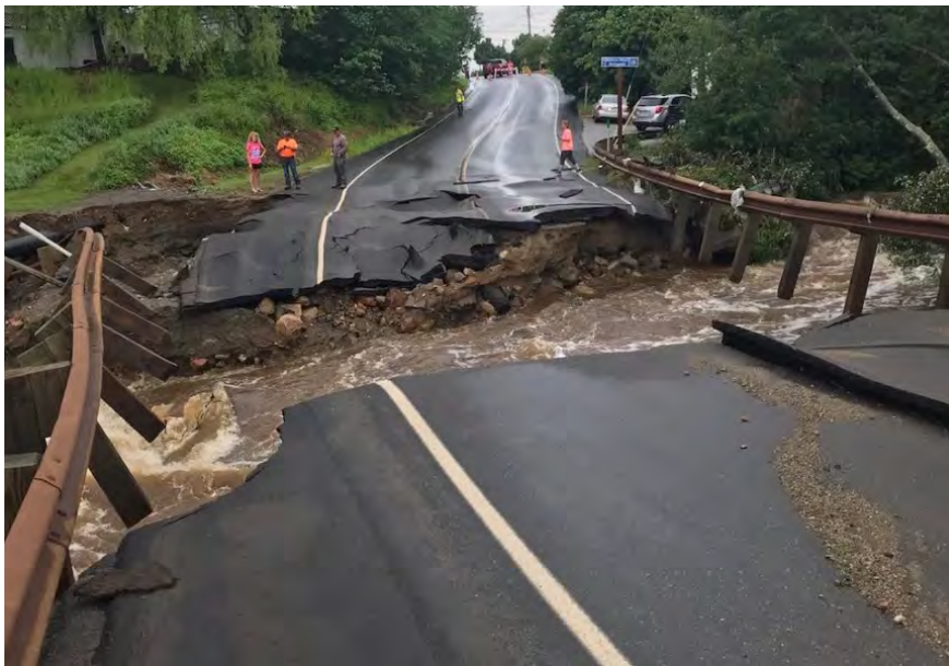
Culverts washed out along Route 186 in the Village of Birch Harbor during a flooding event on June 9, 2021. © Dale Church
